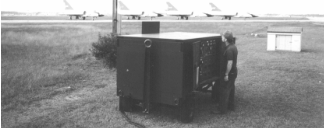
Figure 13: Load bank for adjusting power load on generator
